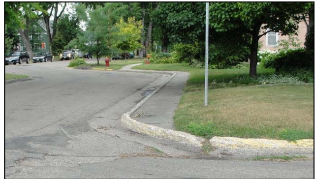
Sidewalk without curb cut, Moorhead
