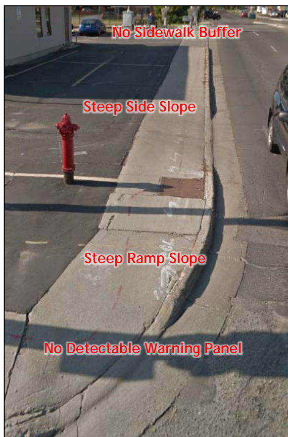
Figure 26 - Example of Pedestrian Deficiencies along 11th Street
