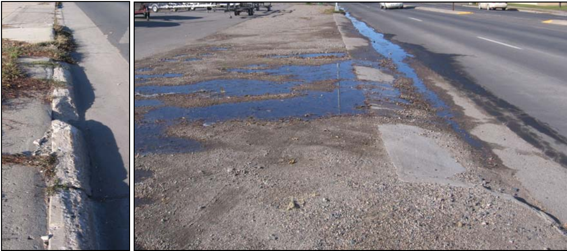
Poor curb and gutter condition, gravel from site affecting function of gutter, and gravel parking area in poor condition.
