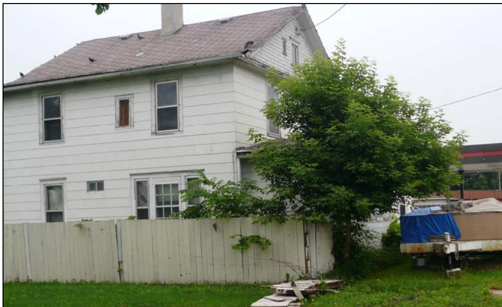
Deteriorating condition of residential property along 1 st Avenue N, combined with prohibited outdoor storage in front yard
